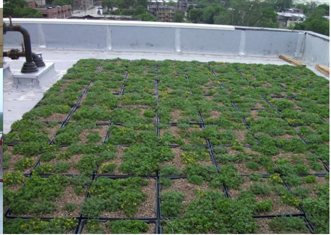
Green Roof Senior Village 2010
