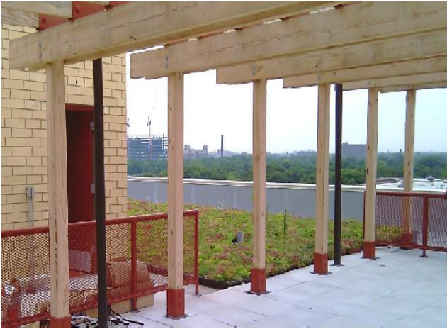
Green Roof Senior Village 2010
